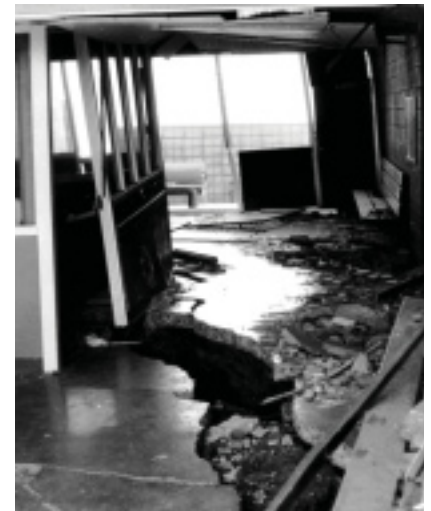
LA County Juvenile Hall, Sylmar, California, damaged by liquefaction during the magnitude 6.6 San Fernando earthquake of February 9, 1971. The broken floor is due to settling of the earth and is not the fault itself. Photo by Jack Meehan, structural engineer.
